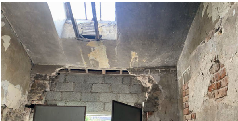
Figure 2-6: Building 3 Repair of Door Head Required
