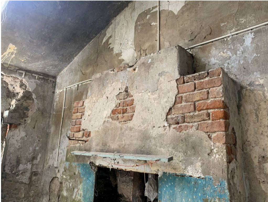
Figure 2-5: Building 3 Internal Finishes in need of repair
