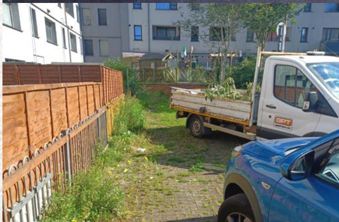
Watergate before works
