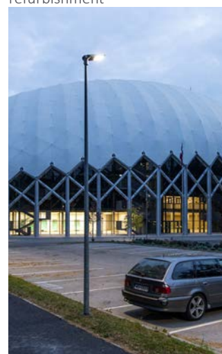
Minimalistic column and luminaire (Credit: Iguzzini)
