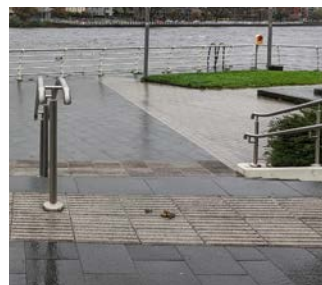
Stainless steel with CHS supports
