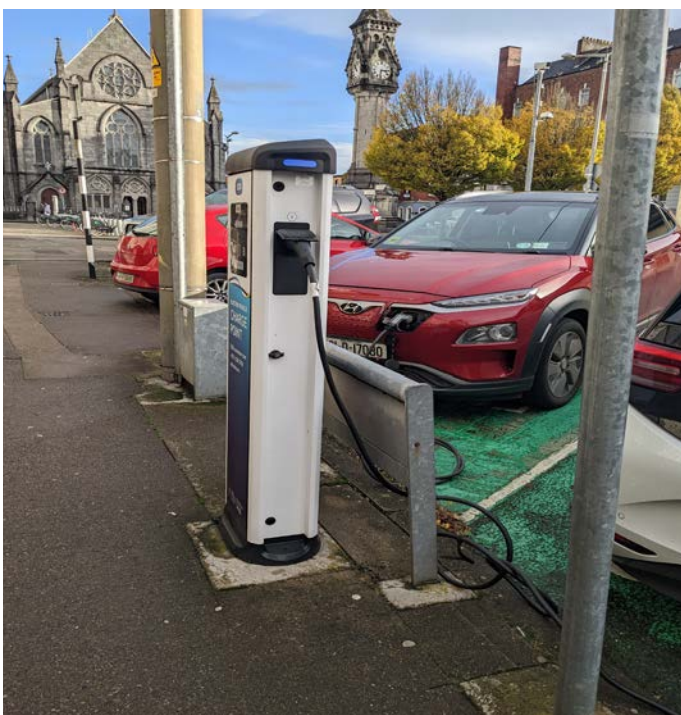
EV charging within Newtown Pery Architectural Conservation Areas
