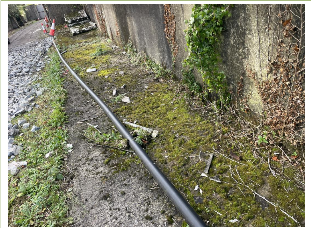
Asbestos cement debris along the rear of building 4
