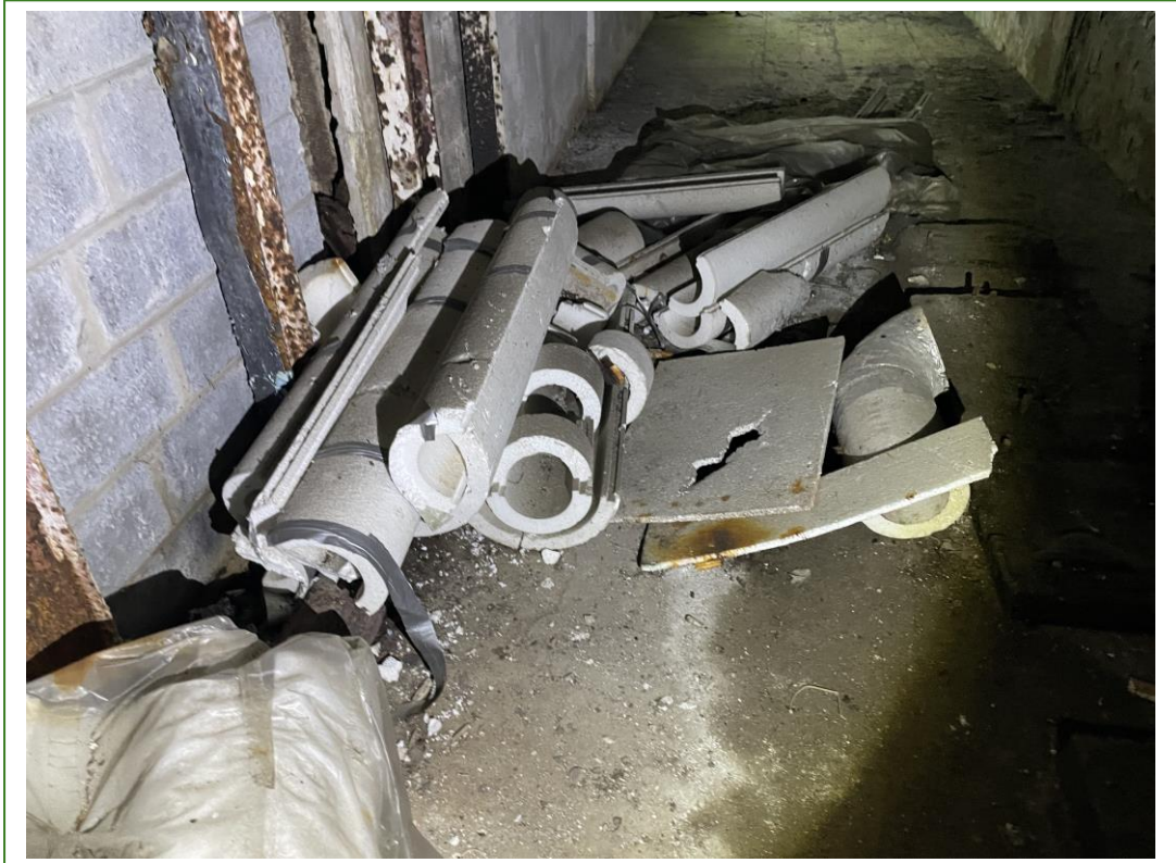
Pipework insulation in building 1
