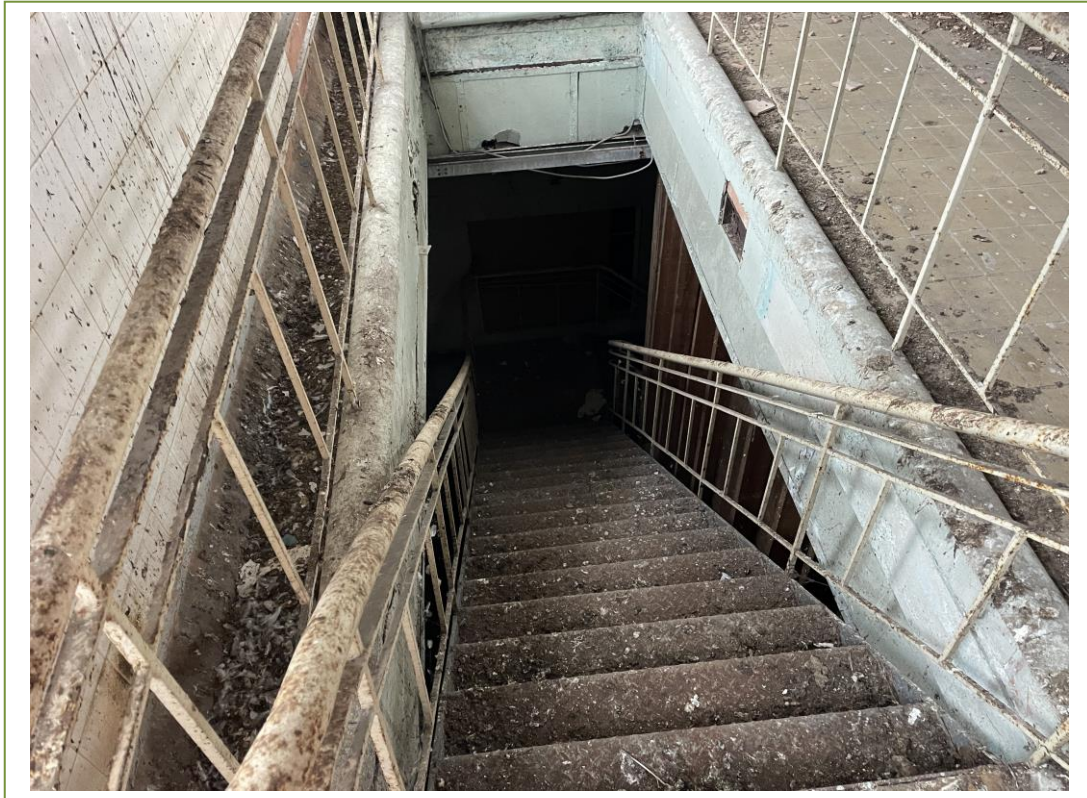
Asbestos insulation board on the walls of the stairs to the 1 st floor in Building 12
