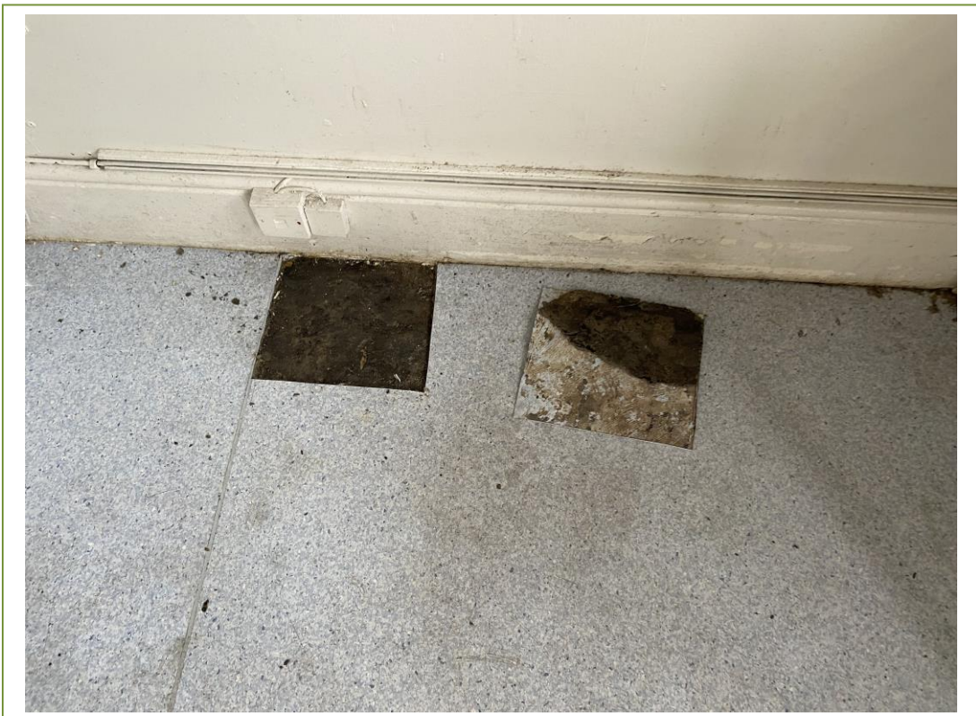
Black compound sampled in the security area of building 10
