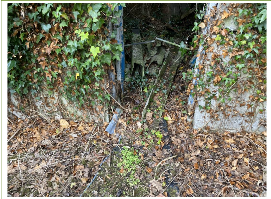
Asbestos cement debris in the rear of Building 17
