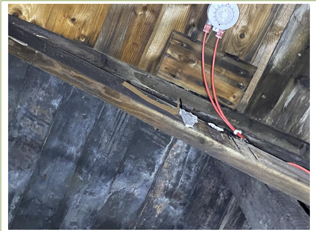
View of the remaining millboard on the higher level of the truss
