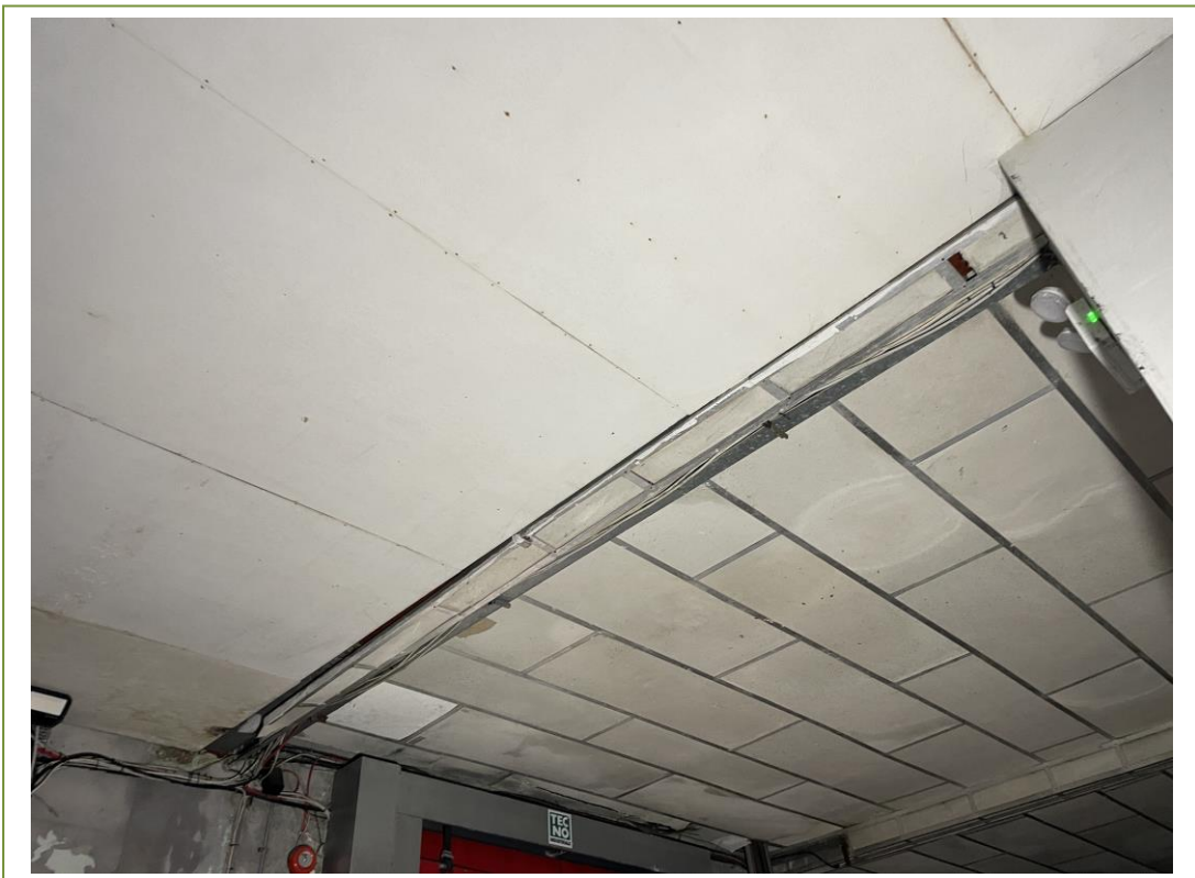
Asbestos insulation board on the ceiling and around the beams in Building 12
