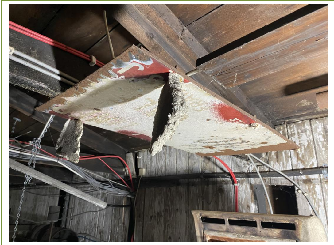
Closeup view of the remaining millboard on one of the panels over the heater
