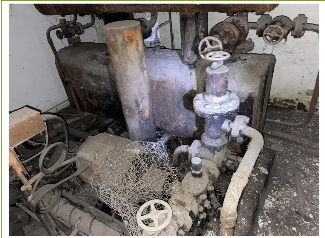
Asbestos containing thermal insulation residue on the boiler unit in the boiler room
