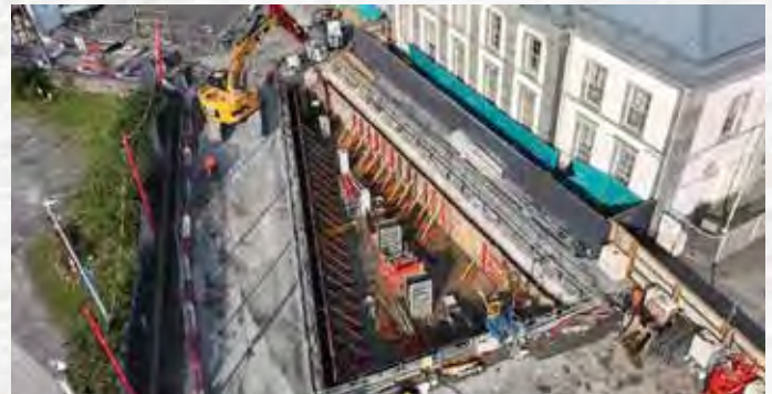
Tidal tank A
