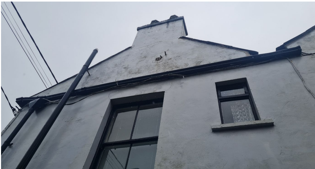
Figure 4: Rainwater goods on the southwest elevation to be renewed.
