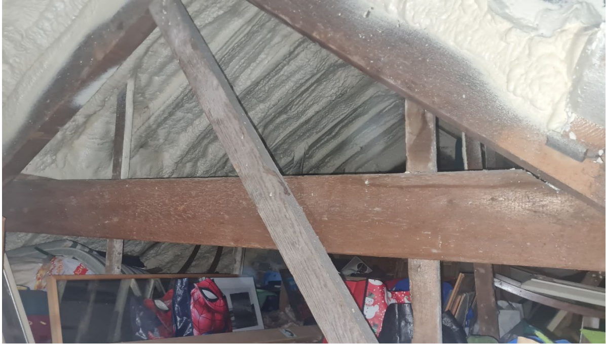
Figure 3: Underside of roof structure to southeast outer slope showing spray foam insulation to be removed.
