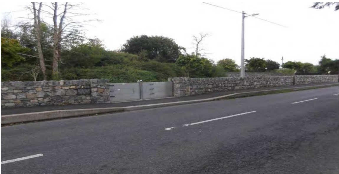
Figure 4-4 Demountable flood defences in Newcastle West (Source: Newcastle West 2014-2020 LAP)
