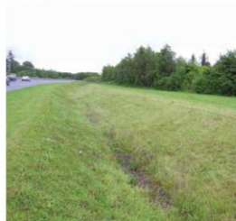
Effectively grassed drains – but wide and mostly dry
