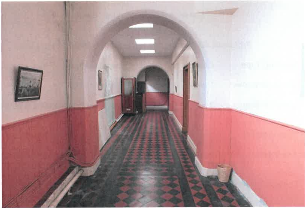
Plate 2020/A(2): View, looking eastwards, of the institutional type corridor that runs in a single storey extension located between the main building and the public road. Note the telephone booth constructed at the top end of the corridor.
