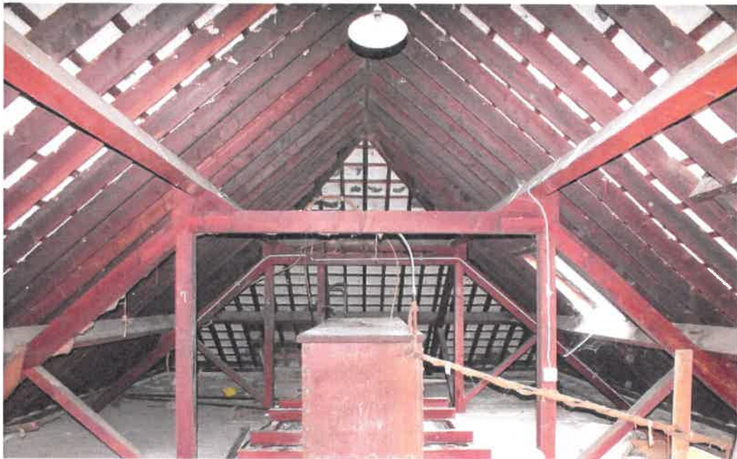
Plate 2020/A(5): An example of the excellent roofing structures that characterise the construction techniques used throughout the various building phases of the Convent Complex's evolution from its foundation through to the completion of the Chapel in the 1950s. Note the white lime plaster beneath the slates. Known as parging, it provided a seal against drafts through the natural slate cover but was also breathable- allowing accumulated moisture in the building to evaporate through.
