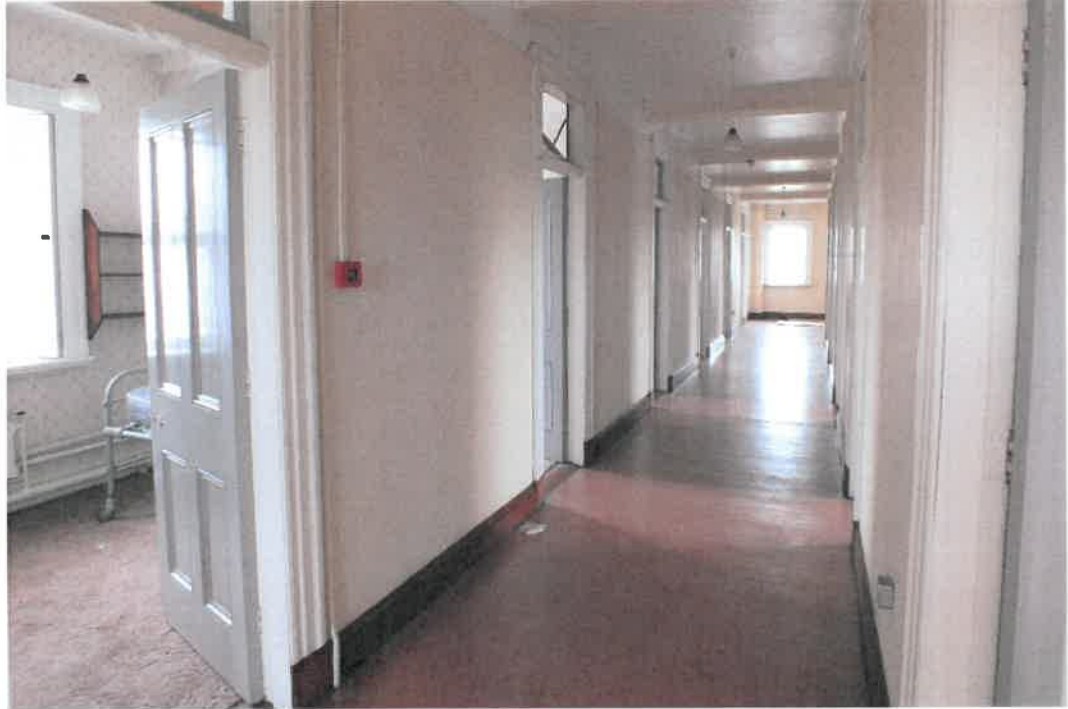
Plate 2020/A(4): One of the many corridors on the second and third floors, off which the individual rooms that provided sleeping accommodation for the members of the Order of Mercy's Community in Doon over many decades.
