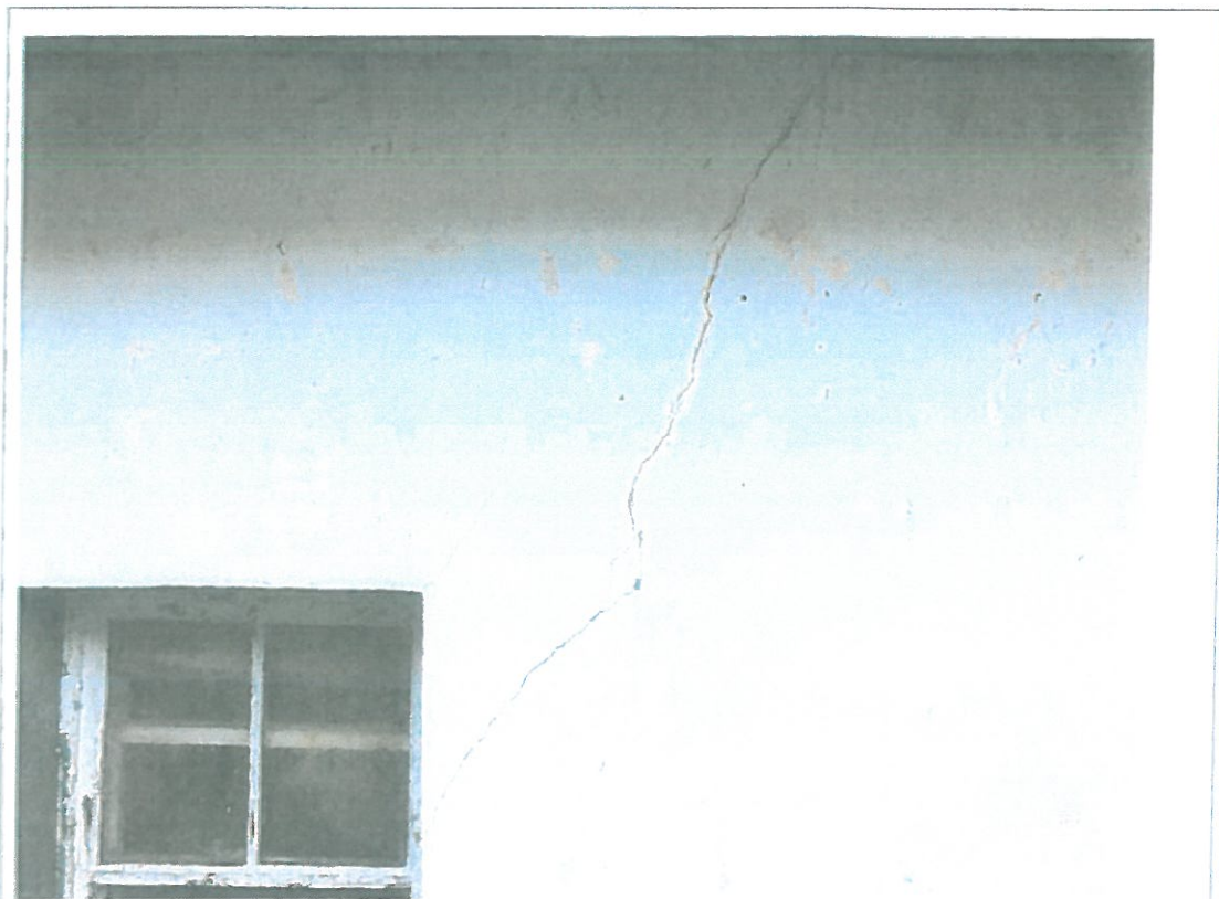
Plate A4: View of another diagonal crack in the rear wall of Quilty's, this one rising from a window opening up towards the eaves level of the house.
