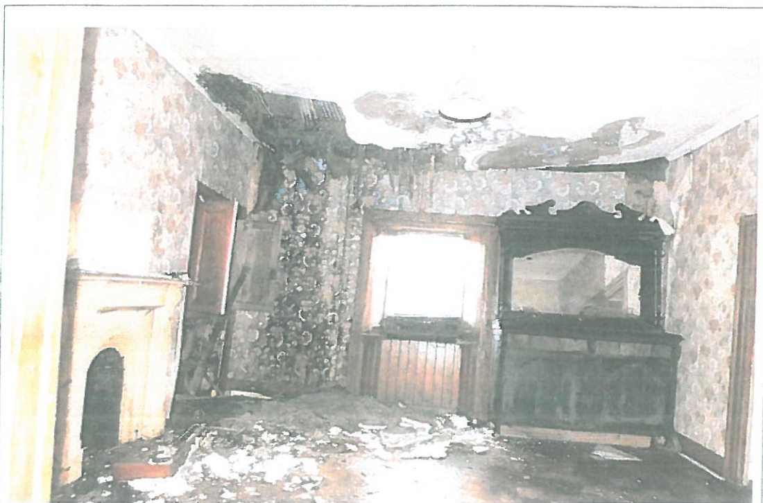
Plate A5: View of the parlour of Quilty's thatched house showing the collapsing ceiling beneath the failed roof and the evidence for rots across the ceiling.
