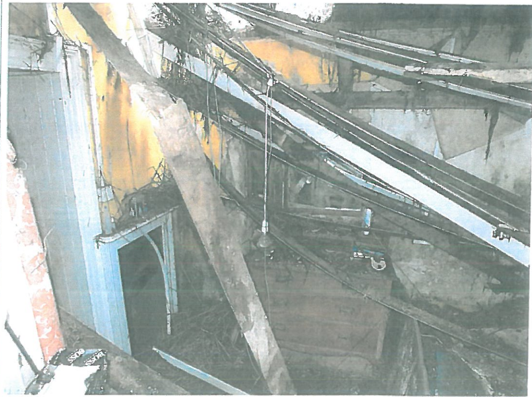
Plate B5: View of the bedroom at the eastern end of Flynn's Thatched House showing the collapsing ceiling beneath the failed roof.
