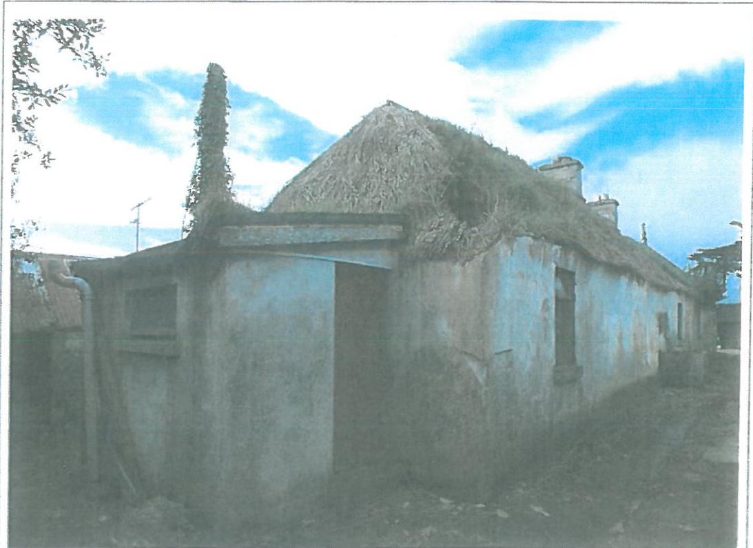
Plate B4: View of the eastern end of Flynn's, from the east-north-east. Note the void in the roofing cover, which has allowed moisture to penetrate with a consequent failure in the timbers forming the hip which have resulted, apparently, in a severe crack occurring on the return.
