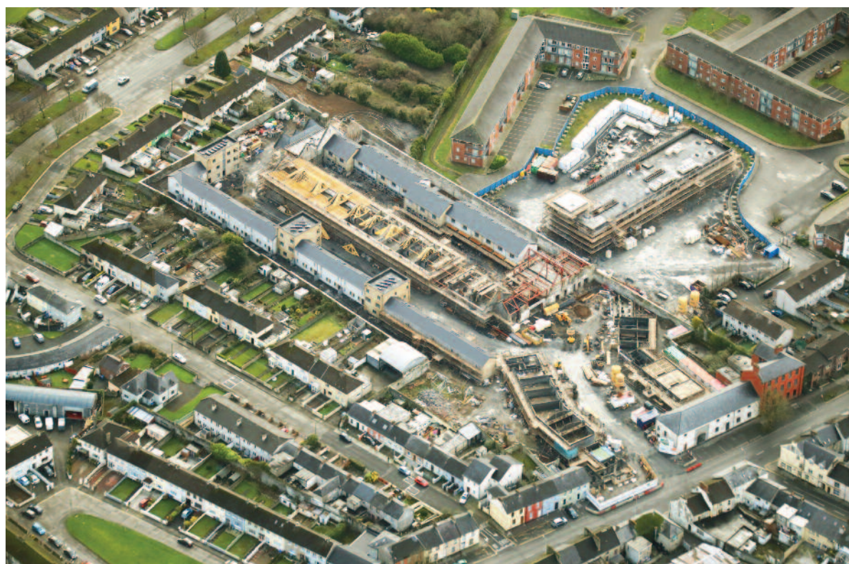
Lord Edward Street site which will deliver 81 housing units, image taken in January 2017
