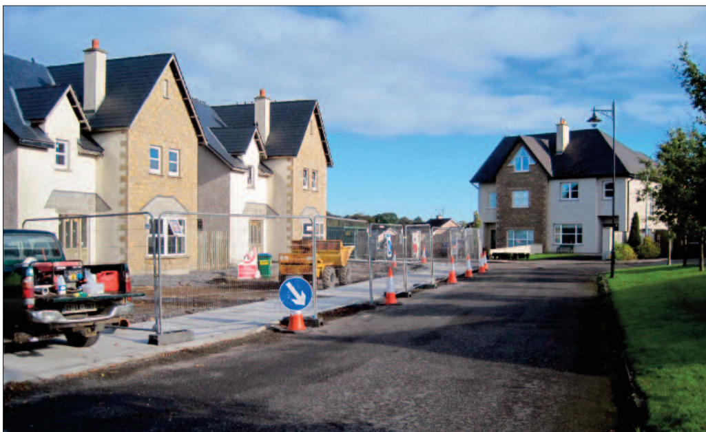
Works ongoing at Bellview, Kilmallock - unfinished Housing Estates
