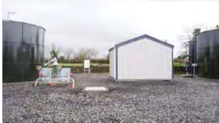
Figure 7.1 Upgraded Treatment Plant at Cappamore
