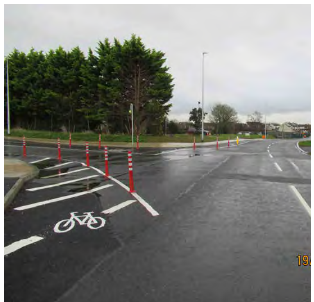
Coonagh Knockalisheen Distributor Road - Cratloe Road Emergency Works
