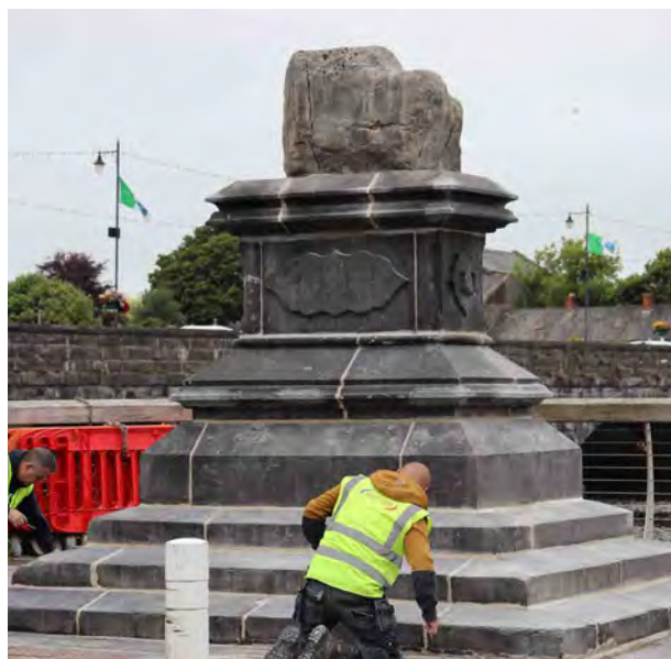
Work in progress, being undertaken by craftsmen from Nolan Conservation, on the Treaty Stone and its surrounds
